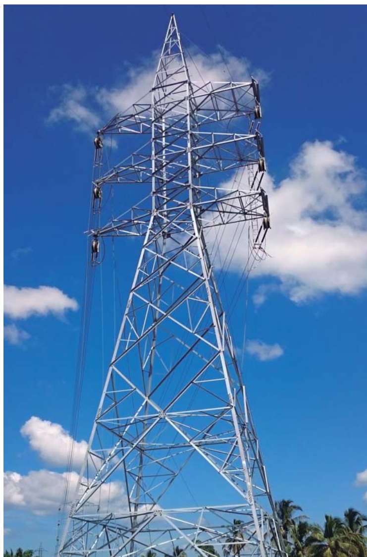
138 kV Santa Catalina-Pizarrete transmission line (Dominican Republic)
