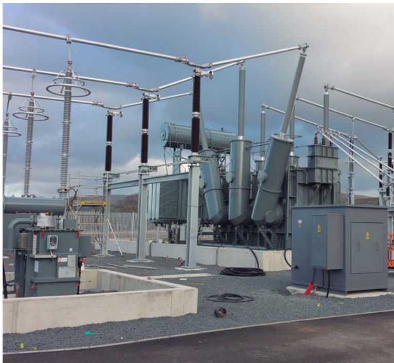
The Hunterston North substation in Scotland (United Kingdom). IQA
