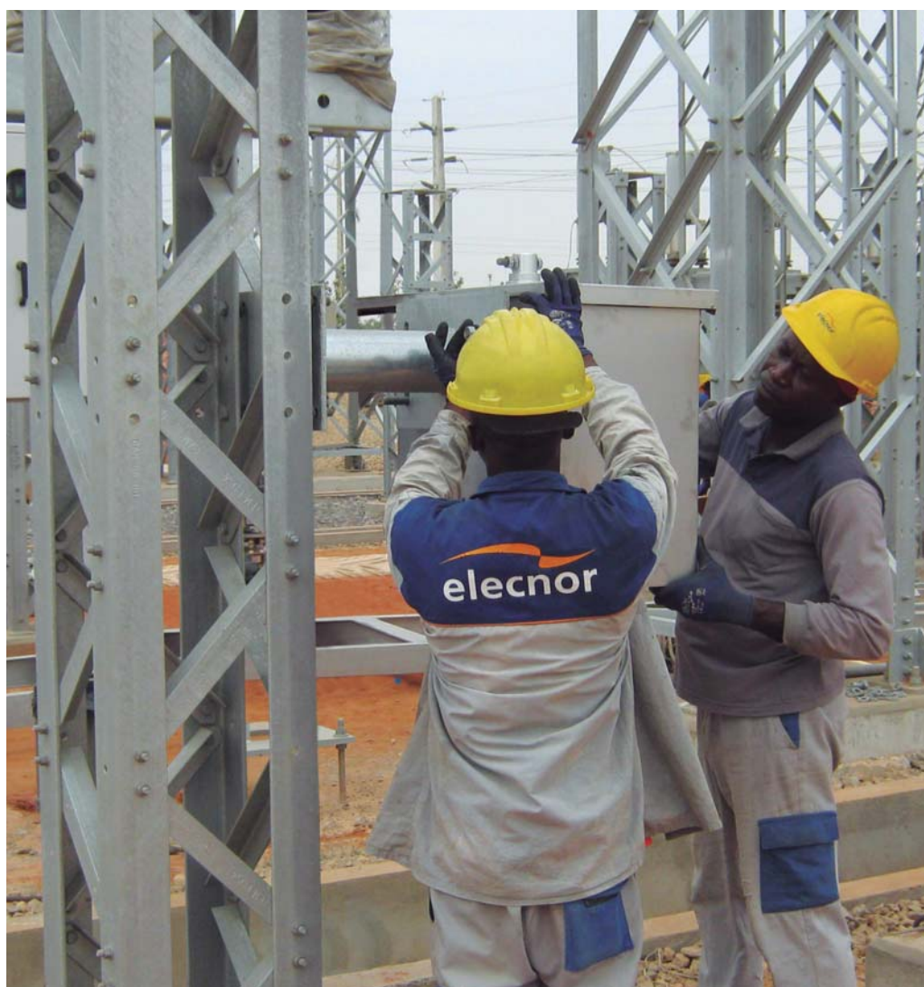
Extension of the 220/60 kV Camama substation (Angola)
