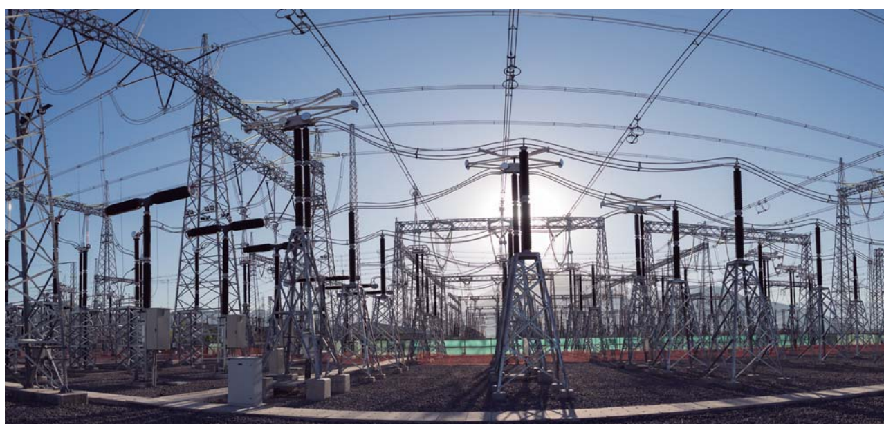
Alto Jahuel 500 kV substation, Chile
