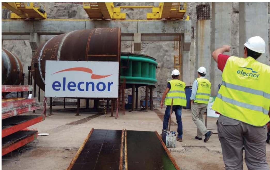
Cambambe 2 hydroelectric plant (Angola)
