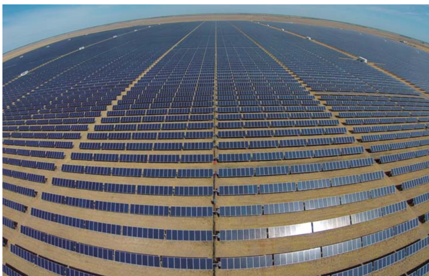
Moree solar photovoltaic plant (Australia)
