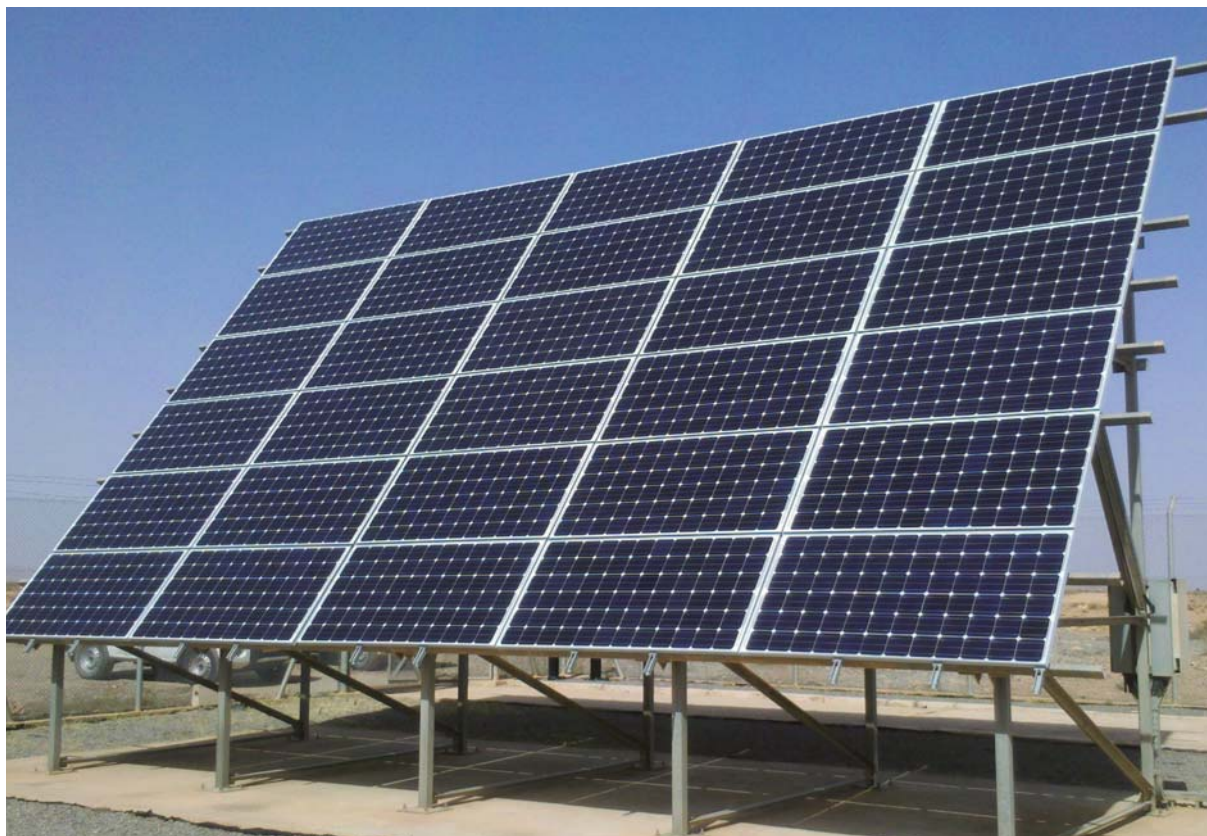
Solar installation for cathodic protection and gas pipeline valve control. Metragaz gas pipeline refurbishment (Morocco)
