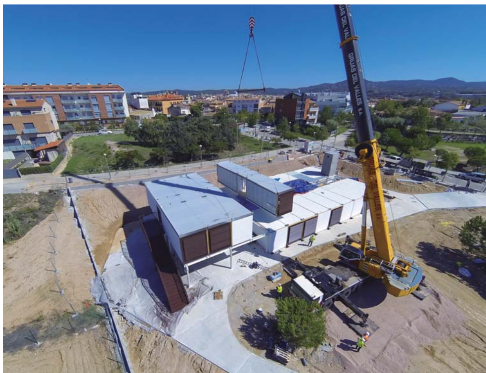
Modular school in Tordera (Barcelona)
