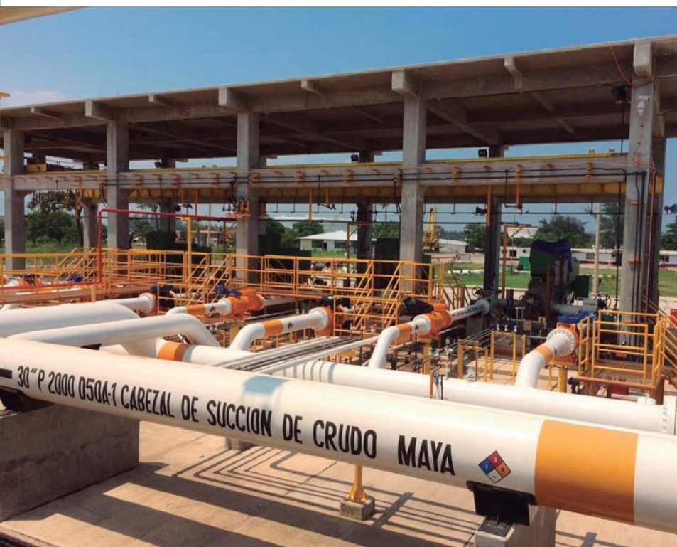
Pump house 4T for transport of crude (Mexico)
